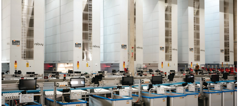
36 newly integrated tray lifts ensure maximum productivity in rebuy's new logistics area.
